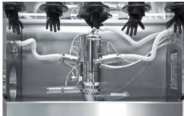
Photo 2: This vacuum conveying system is integrated into a special containment facility for transferring and filling high-potency ingredients and excipients.
